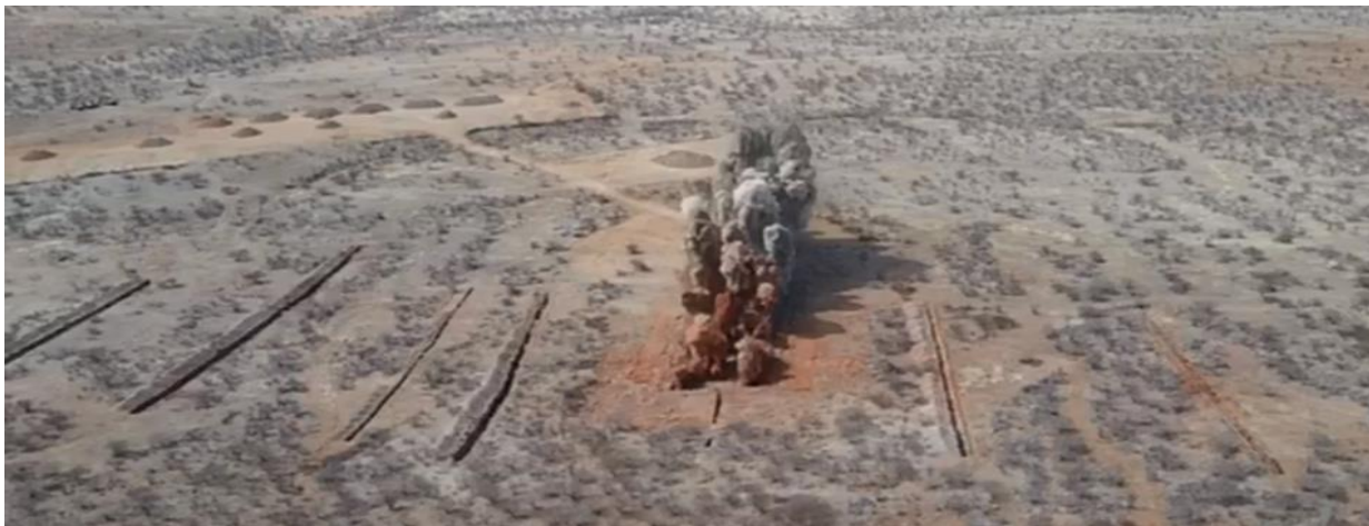
Figure 1: Blast for the bulk sampling pit in central Area 4 deposit at Lofdal by Bulk Mining Explosives (BME); stockpiles in the left background.
